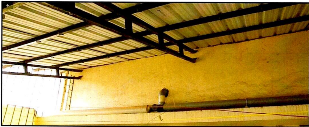
Pipes to carry the harvested rain water to ground level
