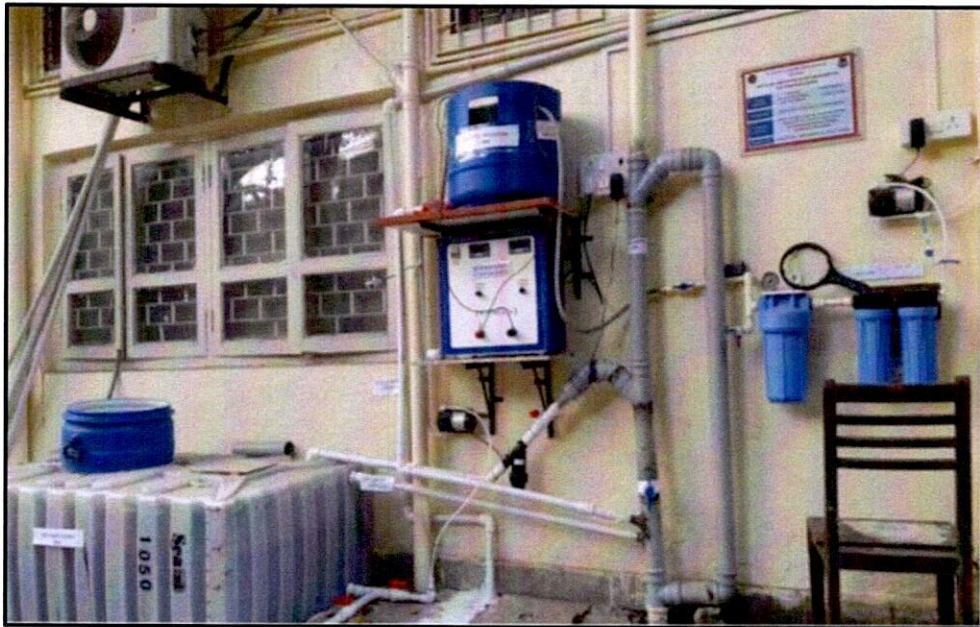
Photograph of the Electrocoagulation Treatment Pilot Plant Site: Back side of Boys' Hostel, St. Xavier's College (Autonomous), Mumbai.
