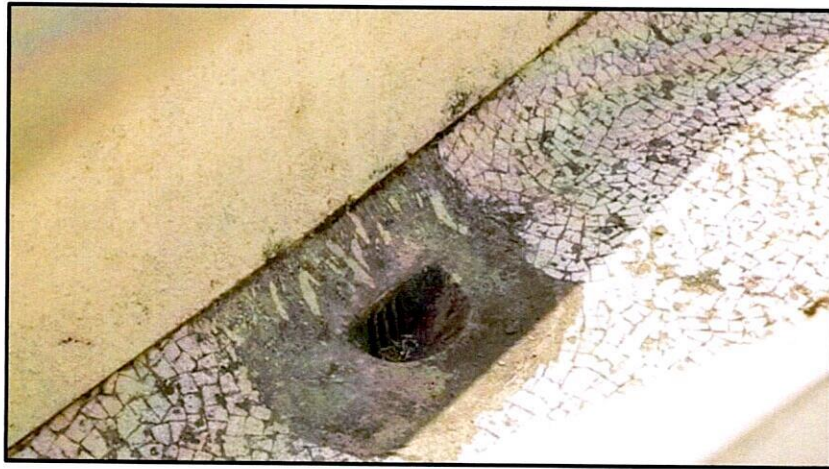
Rooftop drains on the terrace for rainwater harvesting
